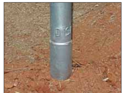
Differential aeration may also be prevented by an additional steel sleeve situated above and below the ground level.
