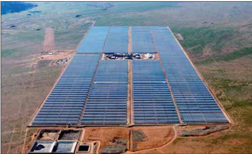
The KaXu plant is using parabolic trough technology. (Power technology)
