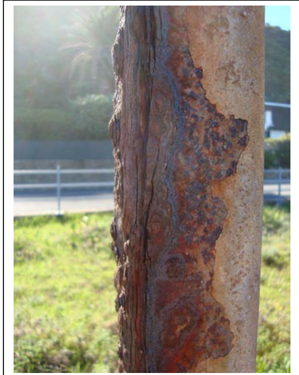
A 2015 close up photograph of the same post showing the advanced state of corrosion to the point where the steel has been perforated
