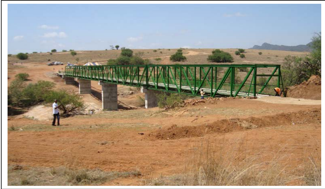
Ntombe River Bridge Hot Dip Galvanized and painted Northern Kwazulu Natal – near the site of the Battle of Ntombe drift 1879
