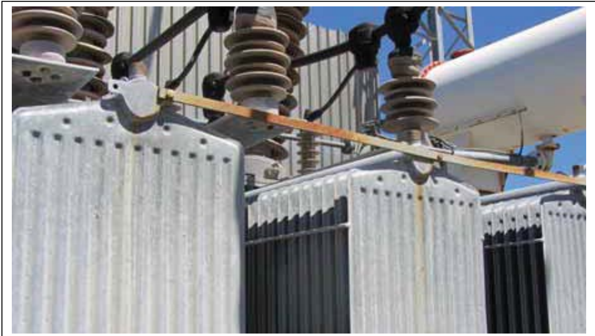
Hot dip galvanized power transformer radiators
