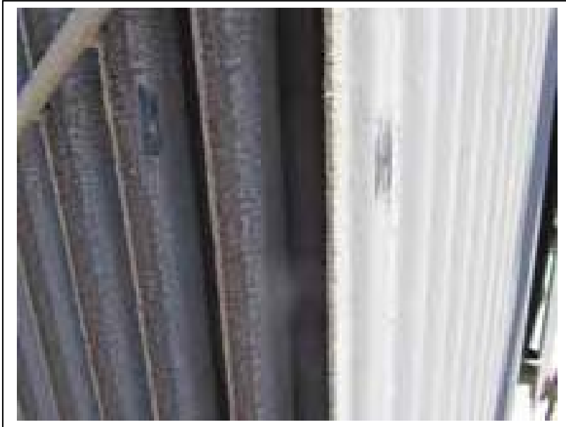
Location the two cleaned area on the transformer radiator showing where residual coating thicknesses were taken
