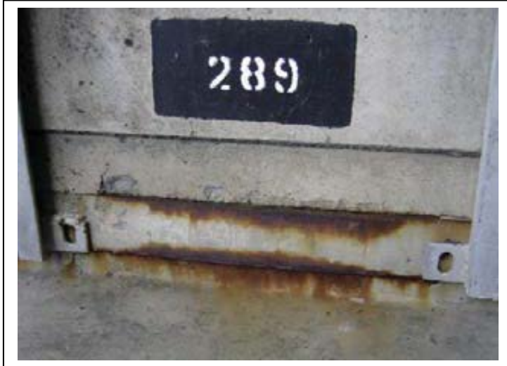
Cast in bottom rail showing the effects of crevice corrosion
