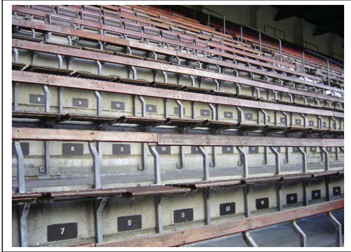
General view of the hot dip galvanized seat support brackets of the Railway Stand
