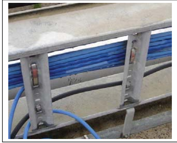
Close up view of the A&S Cable ladder
