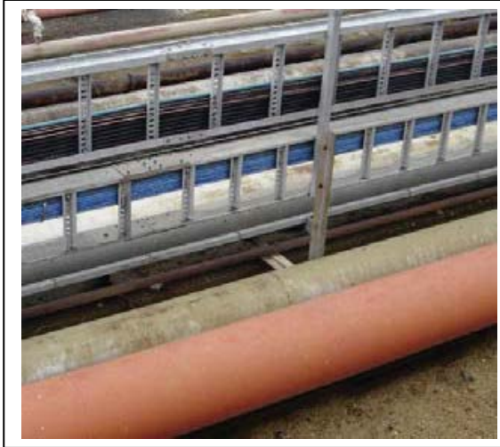
A&S Cable ladder and a more modern edge mounted cable ladder in the background
