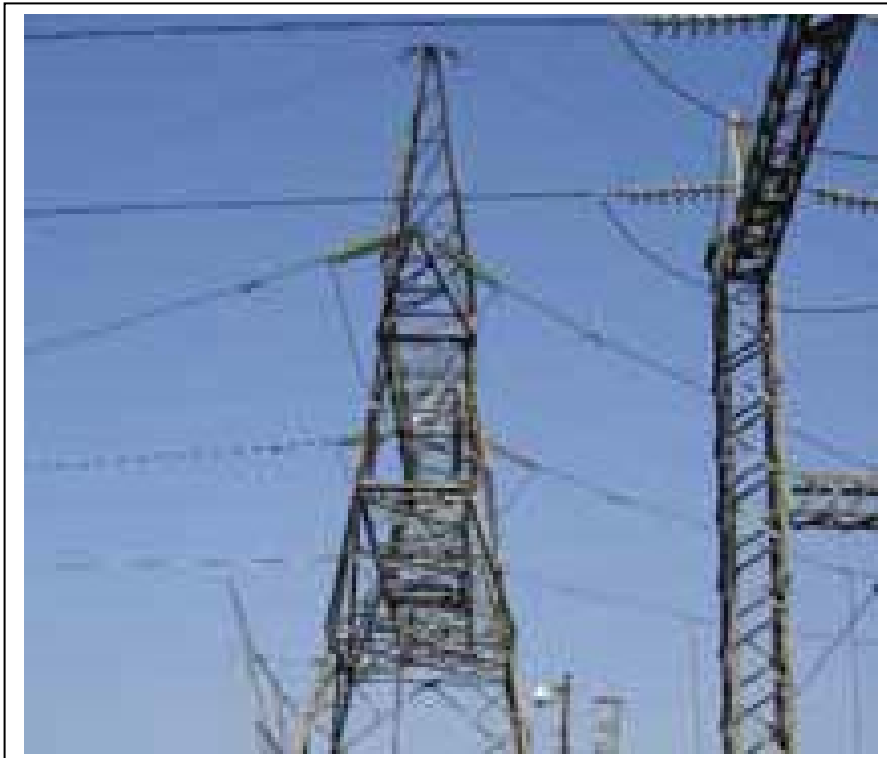
A 132/88kV termination pylon at the Pentrich sub-station of the Georgedale to Pentrich transmission line
