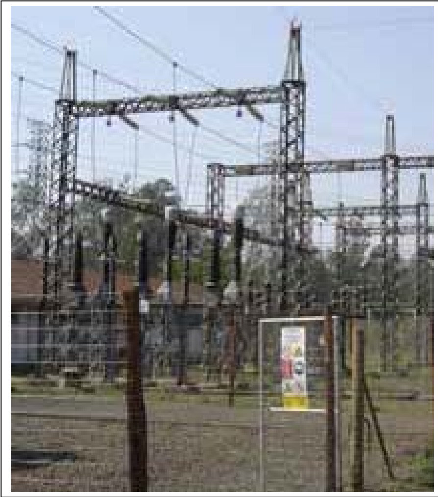
General view of the Pentrich sub-station
