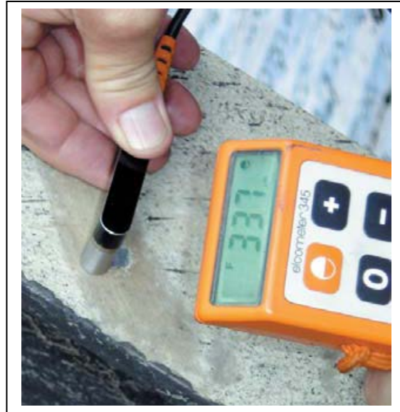
Measurement of the full duplex system (hot dip galvanized plus the top paint system being checked (337µm)
