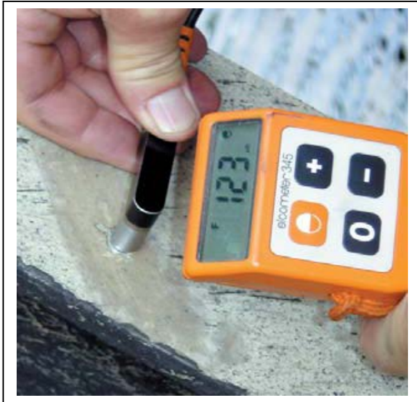
Hot dip galvanized coating being measured (123µm) after the top paint coating had been removed
