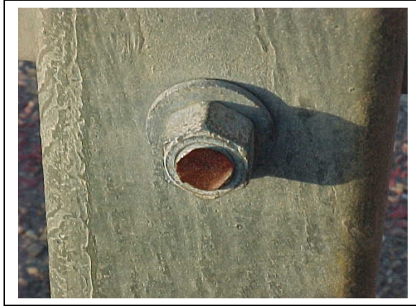
Corroded bolt end cut off after installation; note the absence of under corrosion creep
