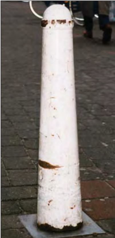
Without a metallic zinc base coat, damage to the powder coating usually results underfilm creep and coating failure.
