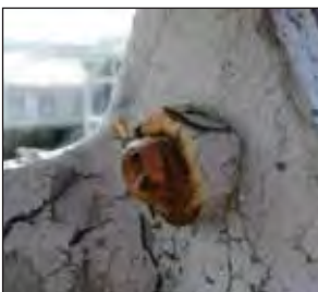
Corroding fasteners will damage the integrity of a structure.
