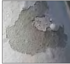
Lack of adhesion due to ineffective surface preparation.
