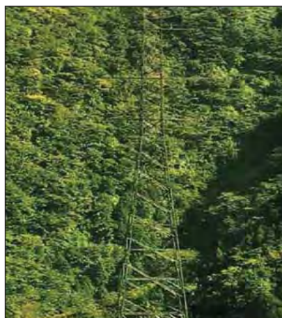
Power transmission tower (galvanized and chemical treatment).
