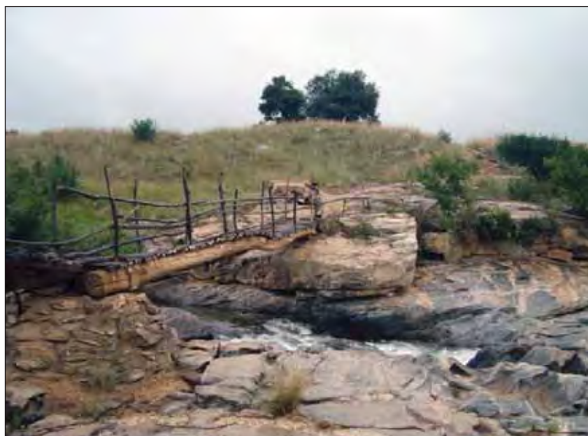
An early rudimentary wooden log bridge over the Ntombe river that served the local community, but ignored any form of safety or construction standards. It was exposed to the elements and incapable of withstanding regular summer flash flooding.
