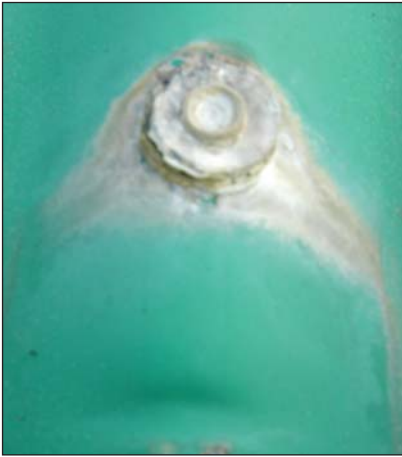
Typical corrosion evident around the majority of the stainless steel screws and aluminium rubber bonded carbon steel washers.
