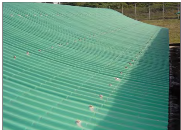
Corrosion products evident around every fastening location.
