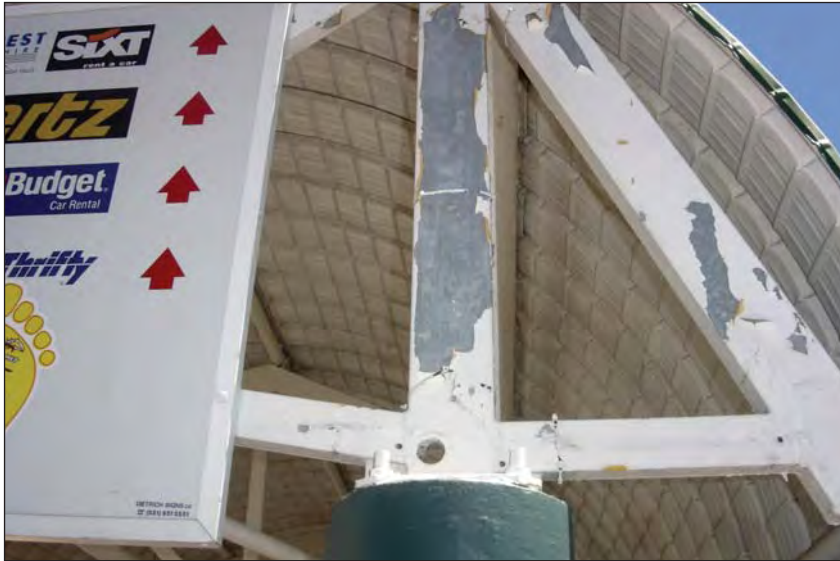
Paint coating delaminating due to little or no zinc surface preparation necessary to accept the mechanically bonded paint coating
