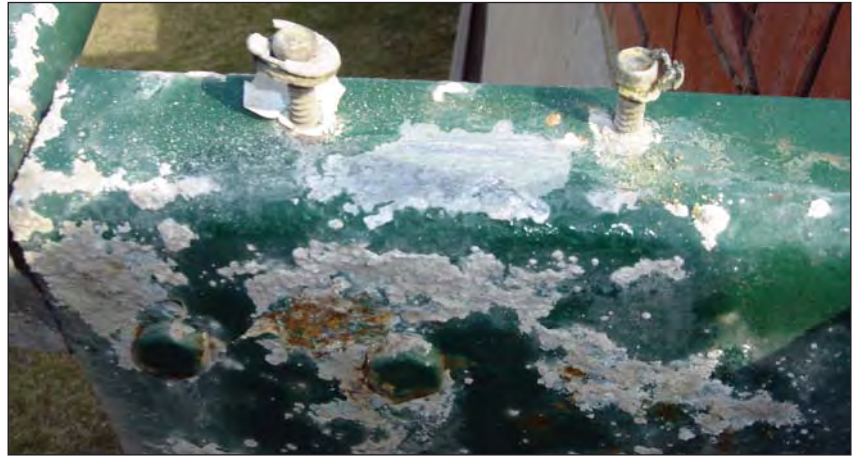
State of the corrosive attack on the hot dip galvanized painted lip channel with remains of the aluminium washers and the relatively "unaffected" stainless steel fasteners.
