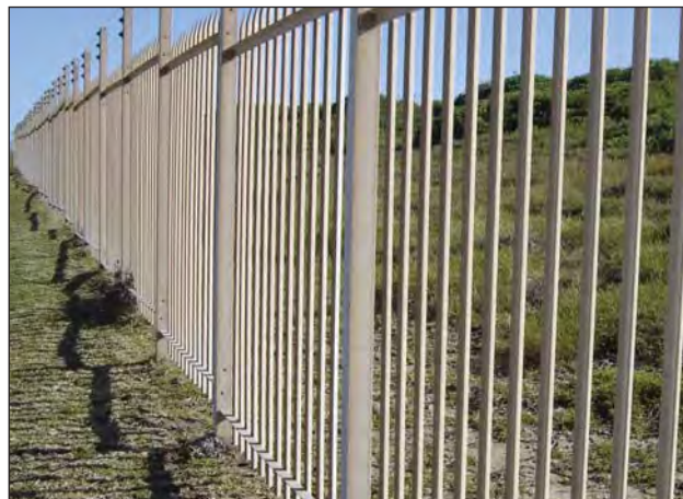
Portion of the perimeter hot dip galvanized fencing.
