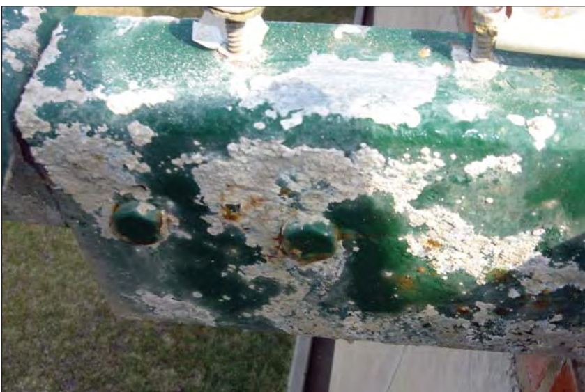
The above two photos show premature coating failures due to incorrect paint used and/or inadequate dry film thickness.
