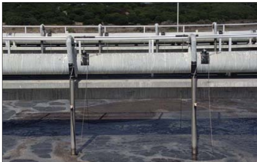
Galvanized pipe facing both the corrosive effects of the effluent and bird excrement!
