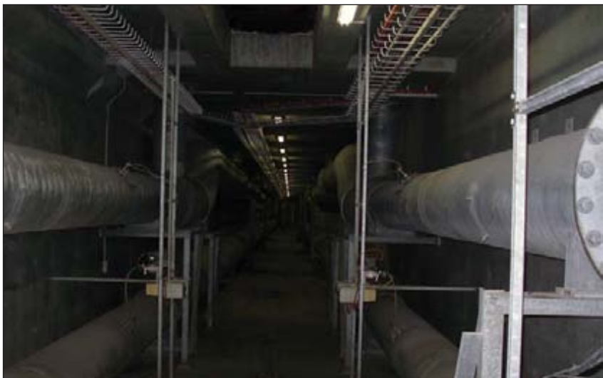
Piping delivering hot air to aeration tanks.
