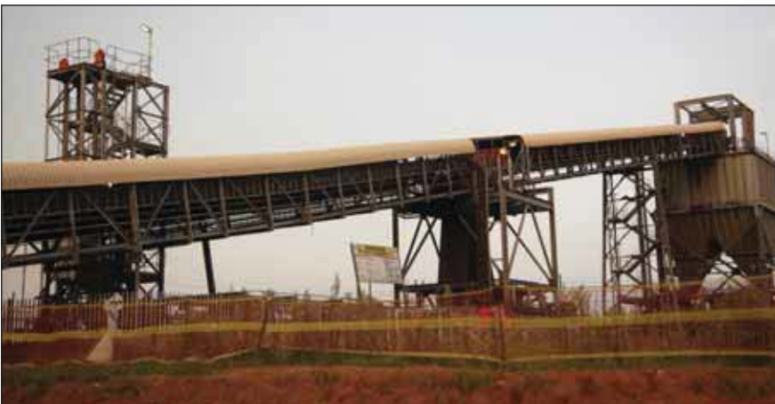
Photos 9 – 11 show 3 views of the Douglas Middelburg Optimisation (DMO) expansion project, including the primary crushing station (top left), 26kms of conveyors (top right) and the Schade Circular Stacker and Portal Stacker Reclaimer (above), completed 2010.
