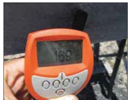
Coating thickness on the structural steel was well in excess of the required 85 \mu m mean. This reading was 169 \mu m.
