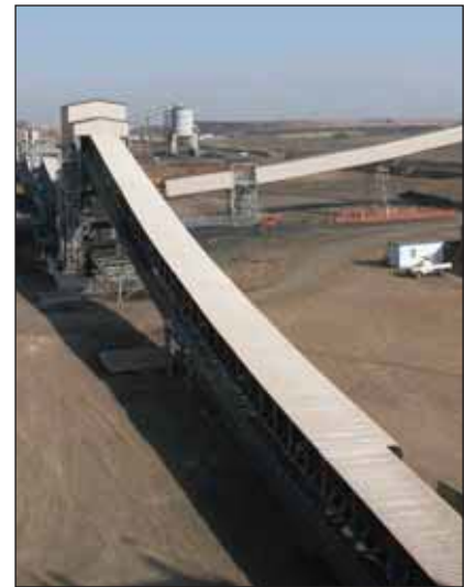
Photo 12 shows a view of the Primary Crushing Station (ROM tip), Rotary Breaker and Plant conveyors at Klipspruit Colliery completed 2009.
