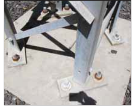
Holding down bolts and nuts.
