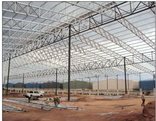
Eureka used Robor's innovative Hybrid Structure for constructing its 11 800m 2 DIY factory in Gauteng. The structural steel is lightweight and allows for customisation.
