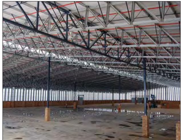
Robor's Hybrid Structures is a cost and time-saving alternative to traditional structural steel systems. The Eureka factory was constructed in just three months.
