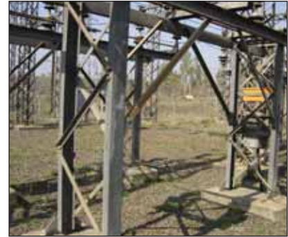
A typical 132/88kV isolator support.
