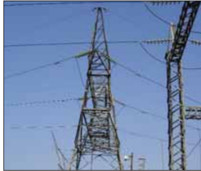
The 132/88kV terminal tower on the Georgedale / Pentrich line.
