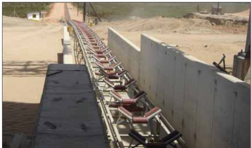
The starting point of the 4km overland hot dip galvanized conveyor that ends at the sea pier from where refined products will be loaded onto sea-barges.
