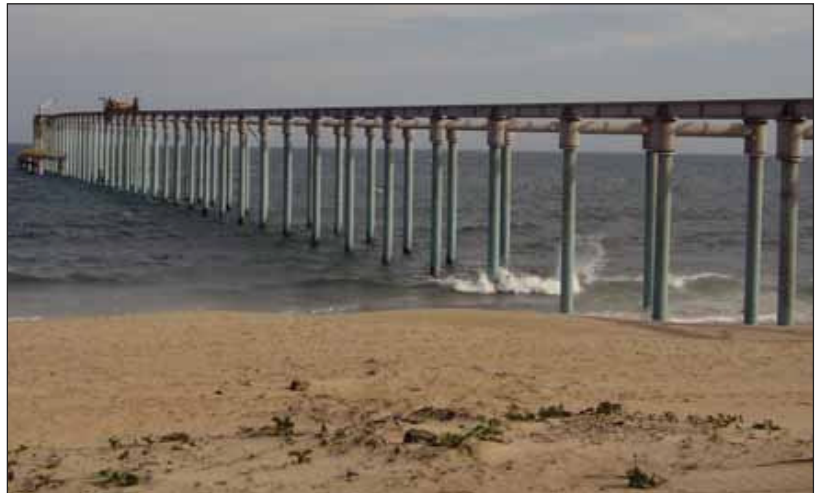
The sea pier and conveyor termination from where refined product will load onto sea-barges for trans-shipment to ships anchored off shore.
