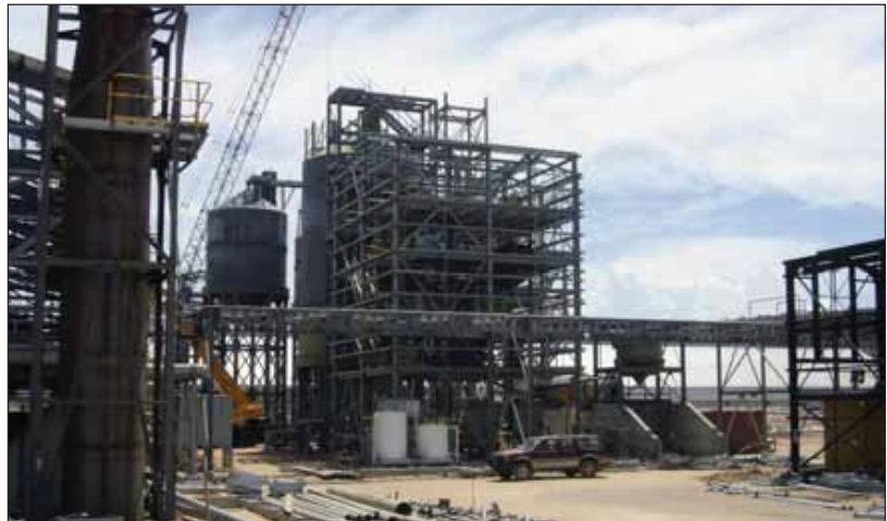
General view of part of the "dry plant" under construction, which will ultimately be used in the refining of titanium products.
