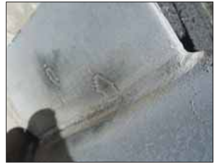
Areas of coating damage (no corrosion creep).
