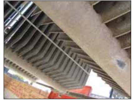
Chloride salts cleaned off the underside of the radiator.
