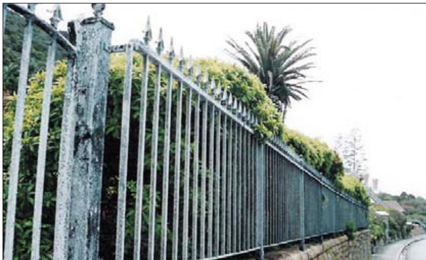
Above and below: An example of a failed duplex coating as a result of insufficient DFT of the paint coating being subjected to the corrosive conditions of Muizenberg. Note the voluminous white zinc corrosion products.
