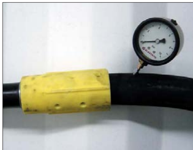
Figure 6: Photo shows the needle valve (not operational) for monitoring correct blast pressure by the operator.
