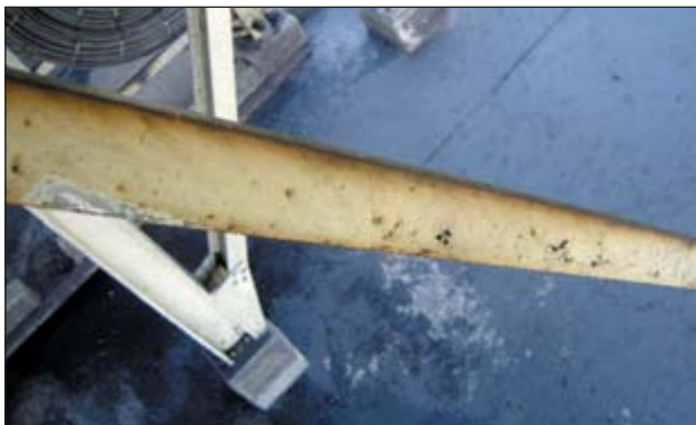
This painted only bracing (no hot dip galvanizing) is showing signs of premature failure amongst the other duplex coated members.
