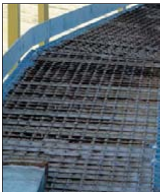
Future maintenance will be required on the hot dip galvanized gratings due to micro climatic conditions.
