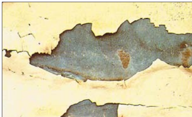
Adhesion failure – paint applied to insufficiently treated hot dip galvanizing.
