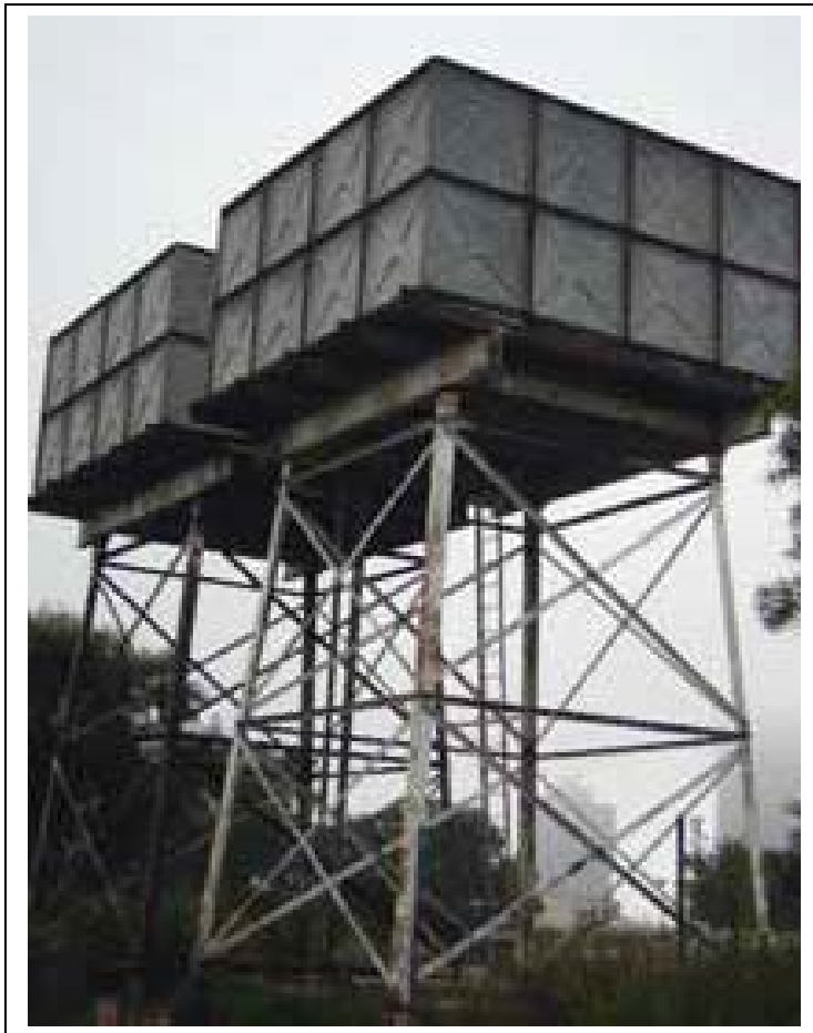
Two “Braithwaite” type tank tanks located on the rampart of the old Johannesburg fort, now the location of the new Constitutional Court of South Africa
