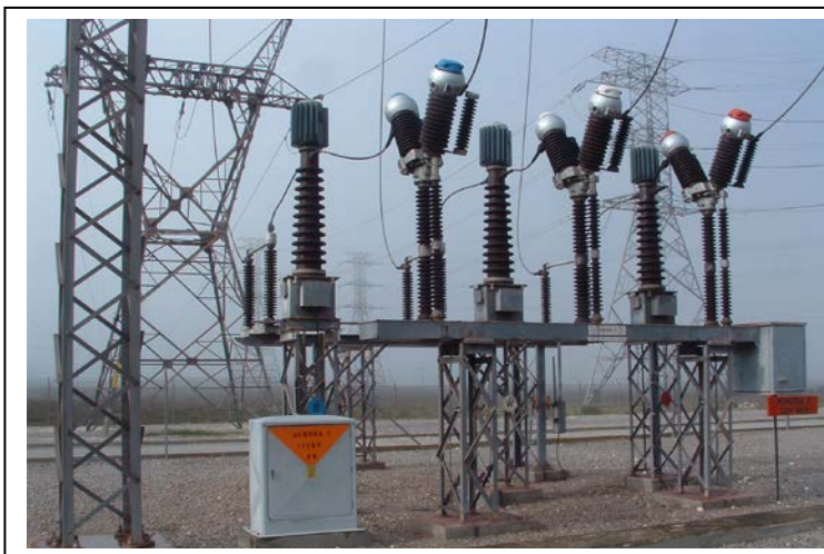
General view of a section of the Blouwater Substation that was inspected on 22 July 2004
