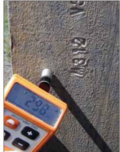
Coating thickness readings taken on the supporting structural steelwork at the access road were still in excess of that required by the specification.
