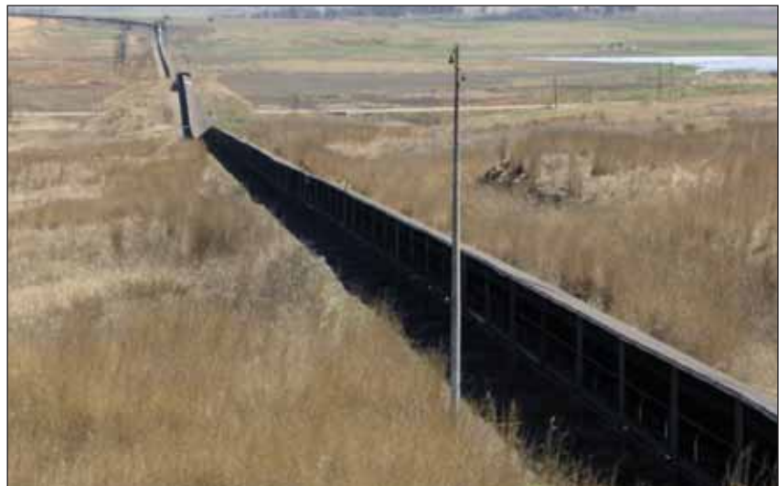
The V3 overland conveyor has been exposed to the elements for in excess of 20 years.
