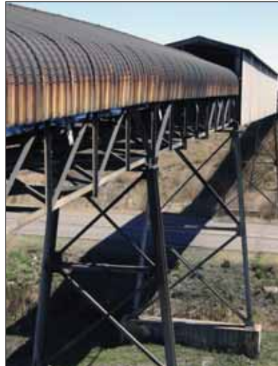
The hot dip galvanized structural steelwork supporting the overland conveyor at an access road, is still performing exceptionally well after 20 years of service.
