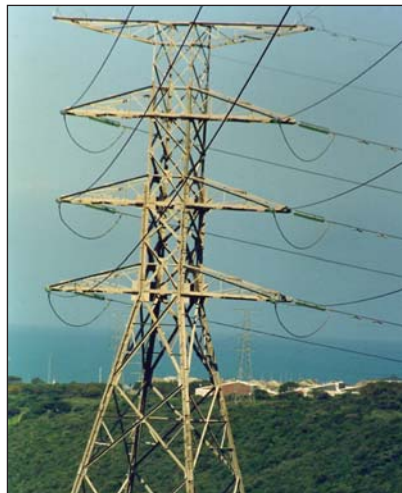
Severe marine coastal conditions. Buffalo-Port Rex Transmission line situated in East London. At the time of the coating inspection, the towers had been in service for about 25 years.
