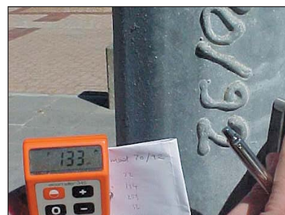
Residual coating thickness (133µm) on the light pole installed in 1992.
