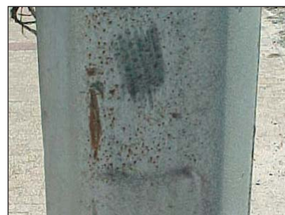
Close-up of the coating on the marine side showing the scraped surface.
