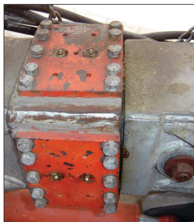
Where hot dip galvanized fasteners were used the comparison to uncoated fasteners is clearly evident.
