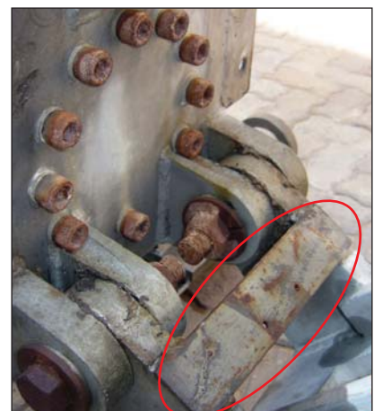
Steel components, added after hot dip galvanizing, were silver painted, again illustrating the corrosive effect relative to the hot dip galvanized surfaces.
