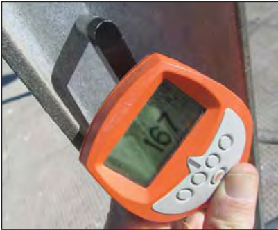
Zinc chlorides salts almost non-existent due to the orientation of the web wrt the direction of the prevailing wind, coating thickness - 167µm.
