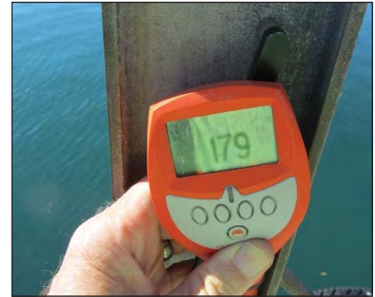
Zinc chlorides salts almost non-existent due to the orientation of the web wrt the direction of the prevailing wind, coating thickness - 179µm.
