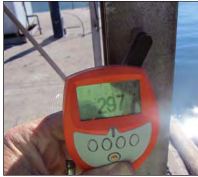
Zinc chloride layer including the hot dip galvanized coating thickness of 297µm.
