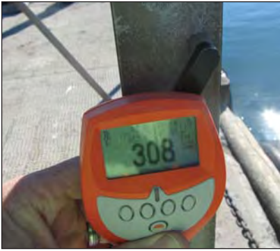
Zinc chloride layer including the hot dip galvanized coating thickness of 308µm.
