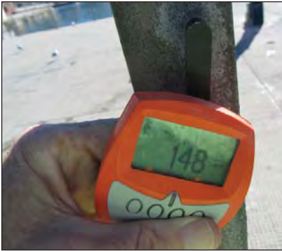
Zinc chloride salts removed and the residual coating thickness measured - 148µm.
