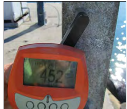
Zinc chloride layer including the hot dip galvanized coating thickness of 452µm.
