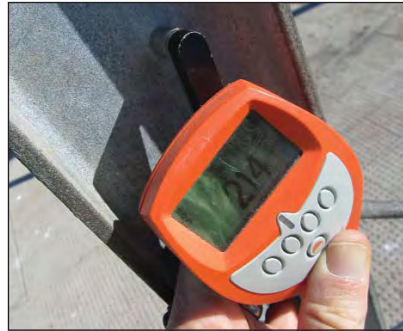
Zinc chlorides salts almost non-existent due to the orientation of the web wrt the direction of the prevailing wind, coating thickness - 214µm.
