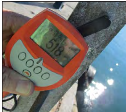
Zinc chloride layer including the hot dip galvanized coating thickness of 518µm.
