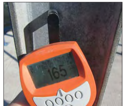
Zinc chlorides salts almost non-existent due to the orientation of the web wrt the direction of the prevailing wind, coating thickness - 165µm.
