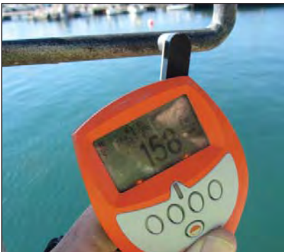
Zinc chlorides salts almost non-existent on round bar climbing hoops, coating thickness - 158µm.
