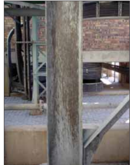
Hot dip galvanized structural steel adjacent to the reagent area.
