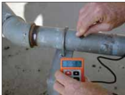
Coating thickness of a hot dip galvanized water pipe in the reagent area.
