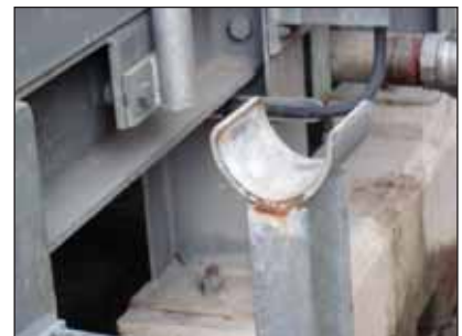
Coating damage and inadequate repair in the reagent loading area.
