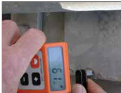
Coating thickness at damaged area in reagent loading area (#1).
