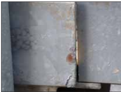
Damaged coating in reagent loading area.
