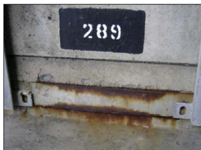
View of cast in non-galvanized bottom rail showing corrosion products.
