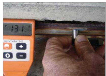
Corrosion products removed and residual coating thickness (13.1 \mu m) taken on bottom rail.
