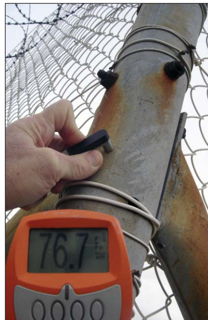
Photo left, shows the residual hot dip galvanized coating thickness on the boundary fence corner post.
