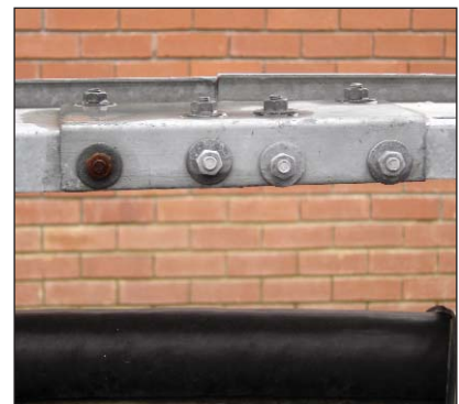
Only zinc electroplated fasteners have been supplied in some instances.
