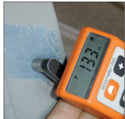
Total coating thickness reading on the cleaned up side rail of the cable ladder.
