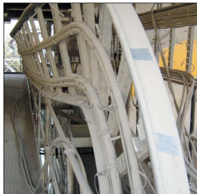
Insitu cable ladders in the redundant Transfer Station No. 1.
