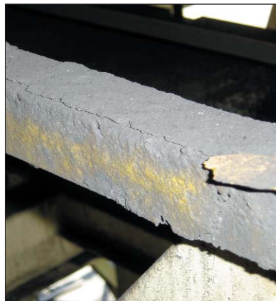
In comparison the paint coating on the carbon steel handrails has failed.
