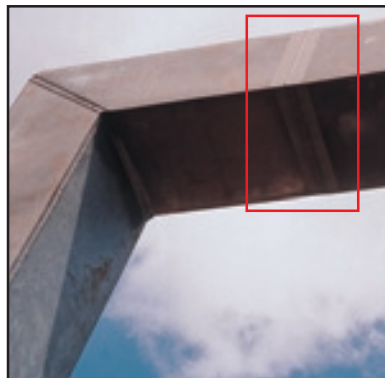
Figure 110. Site welded joint on hot dip galvanized highway sign gantry - repaired by "Zincfix".
