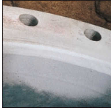
Figure 109. Zinc metal spray applied to a small uncoated area on a pipe section, adjacent to the flange.
