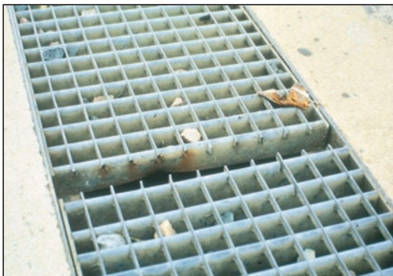
Figure 92. After 20 years of marine exposure, this site cut unrepaired hot dip galvanized steel grating still offers cathodic protection at the cut ends.
