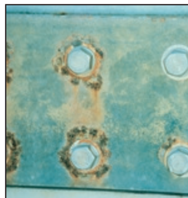
Figure 94. Stainless steel fasteners attached to hot dip galvanized plate in immersed conditions, note the sacrificial attack of the zinc coating surrounding uninsulated fasteners compared with the insulated fastener where no attack of the surrounding zinc has taken place.
