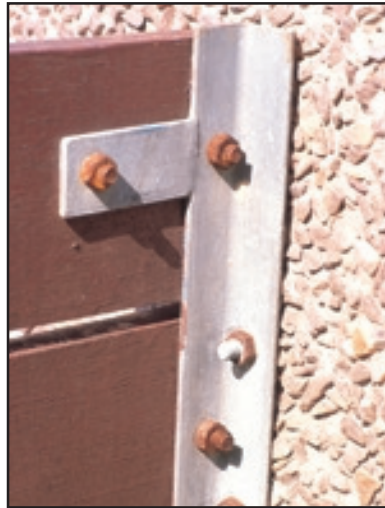
Figure 101. An assortment of zinc coated bolts showing the importance of coating thickness in a particular environment.
