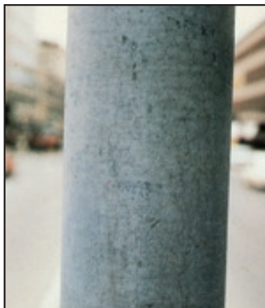
Figure 85. Exposed surface of a hot dip galvanized coating with outer layer of pure zinc. The shiny surface disappears to be replaced by grey corrosion products (sometimes called zinc patina).
