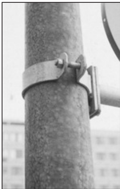
Figure 87. Discoloured surface on lighting column. Coating consists mainly of an iron/zinc alloy that grows out to the surface. Iron is freed during corrosion, which leads to rust formation. It is only surface rust and is of aesthetic significance only. The bracket for the traffic sign has a coating of pure zinc as an outer layer.
