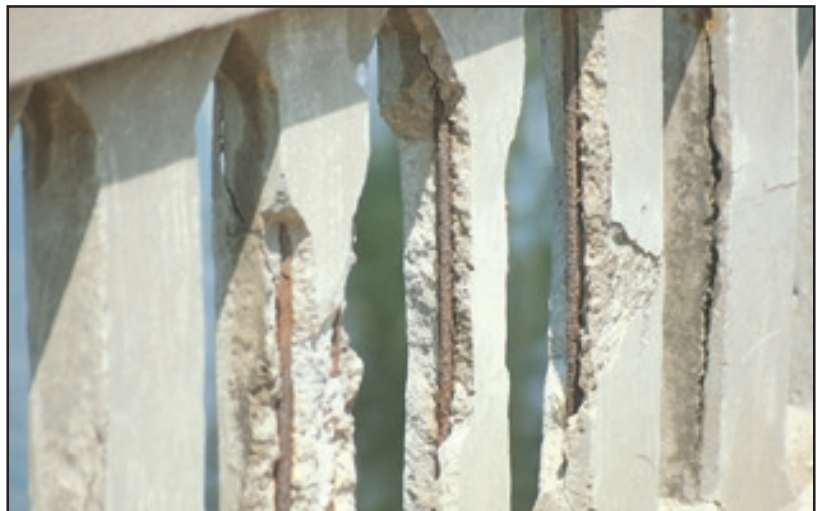
Figure 99. Spalling of the concrete layer on reinforcing steel in a concrete bridge balustrade.
