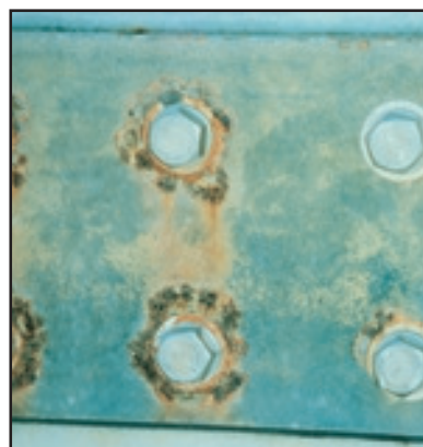
Figure 94. Stainless steel fasteners attached to hot dip galvanized plate in immersed conditions, note the sacrificial attack of the zinc coating surrounding uninsulated fasteners compared with the insulated fastener where no attack of the surrounding zinc has taken place.
