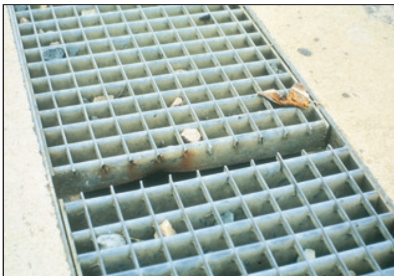
Figure 92. After 20 years of marine exposure, this site cut unrepaired hot dip galvanized steel grating still offers cathodic protection at the cut ends.
