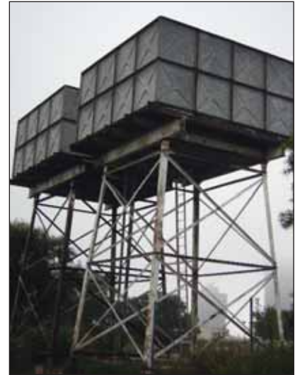
General view of water tanks.
