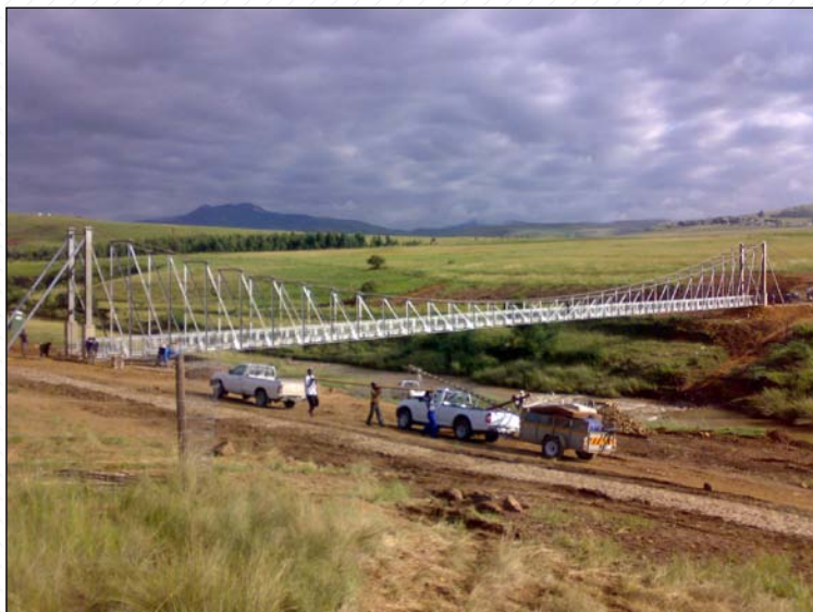
The crew finishing up after a successful day on site at the almost completed Bisi Pedestrian Bridge.
